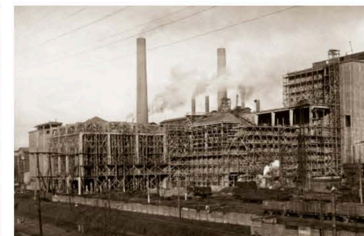
Budowa rozdzielni 110 kV, rozbudowa hali maszyn i budowa kotłowni 80 atmosfer – 1944 r. / Construction of a 110 kV switching station, expansion of the engine house and construction of 80 atm boiler house – 1944
